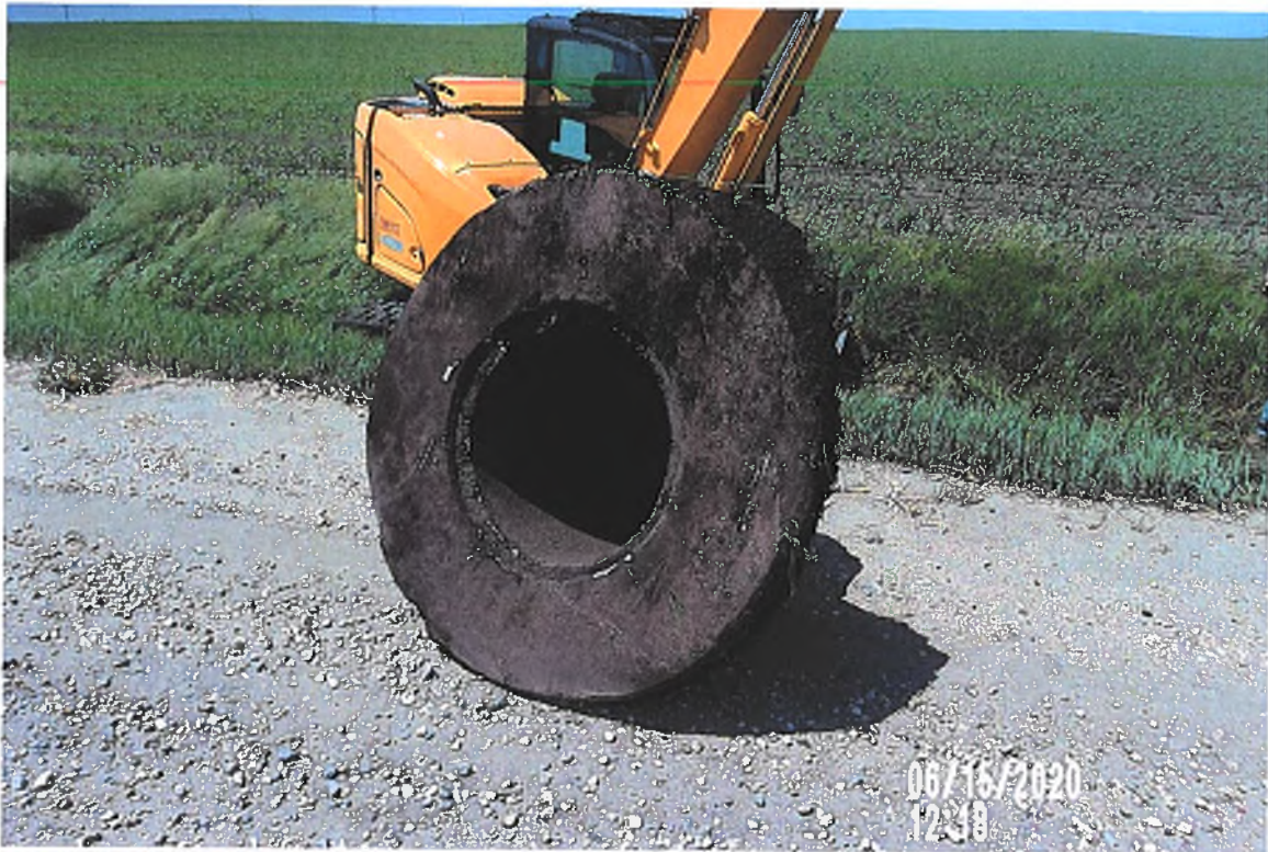
PICTURE # 3748 SHOWING 24" BEEHIVE INTAKE REMOVED 656'± NORTH OF HWY DLS ON WESTSIDE OF AA AVE.
