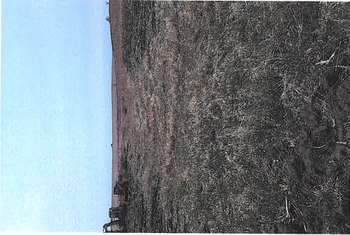
PICTURE #8 IS LOOKING SOUTH AT GRASS WATERWAY NORTH OF 36" CMP SURFACE DRAIN INLET
