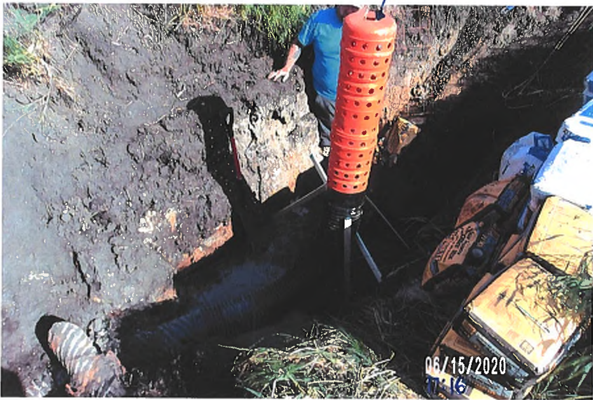
PICTURE # 3758 IS LOOKING SE SHOWING 8" HICKEN BOTTOM SUPPORTED UP BEFORE CONCRETE POURED. GPS 1212 TOP 8" HICKEN BOTTOM
