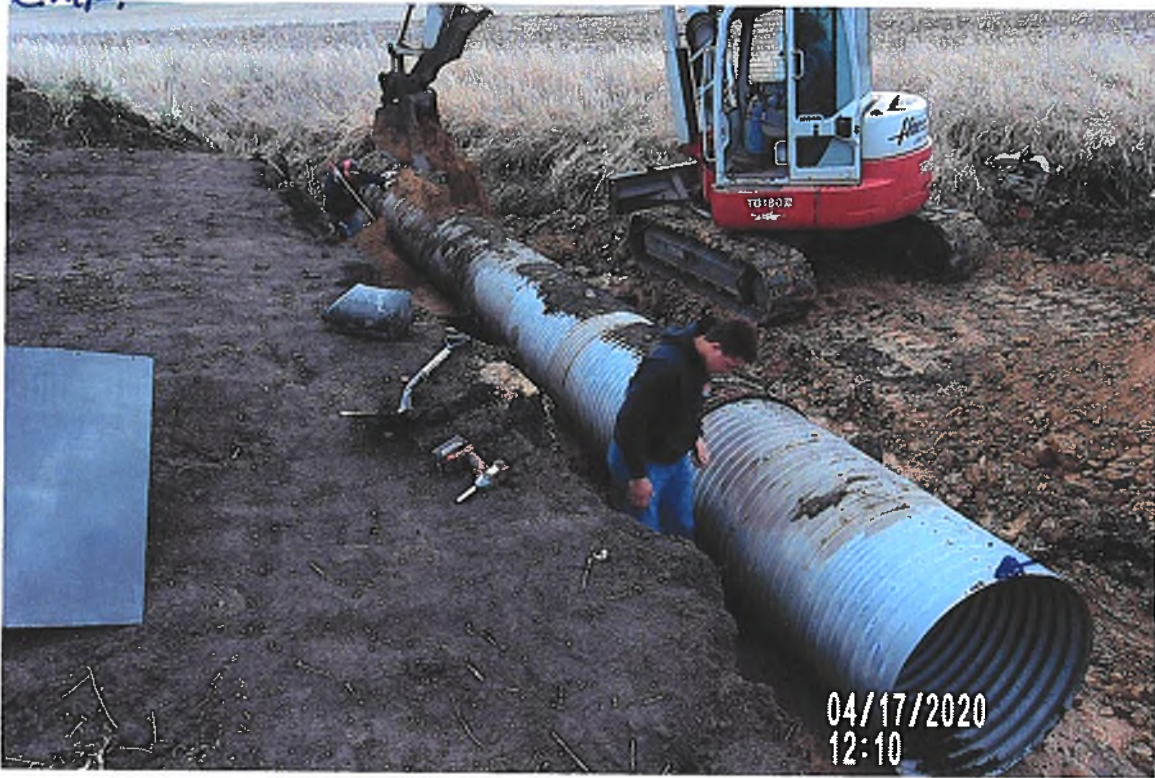
PICTURE #3379 IS LOOKING SW SHOWING 36" CMP SURFACE DRAIN SET IN PLACE WITH CREW BACKFILLING LIMY CLAY AROUND SURFACE DRAIN AND TAMPING SOIL UNDER HAUNCH OF CMP.
