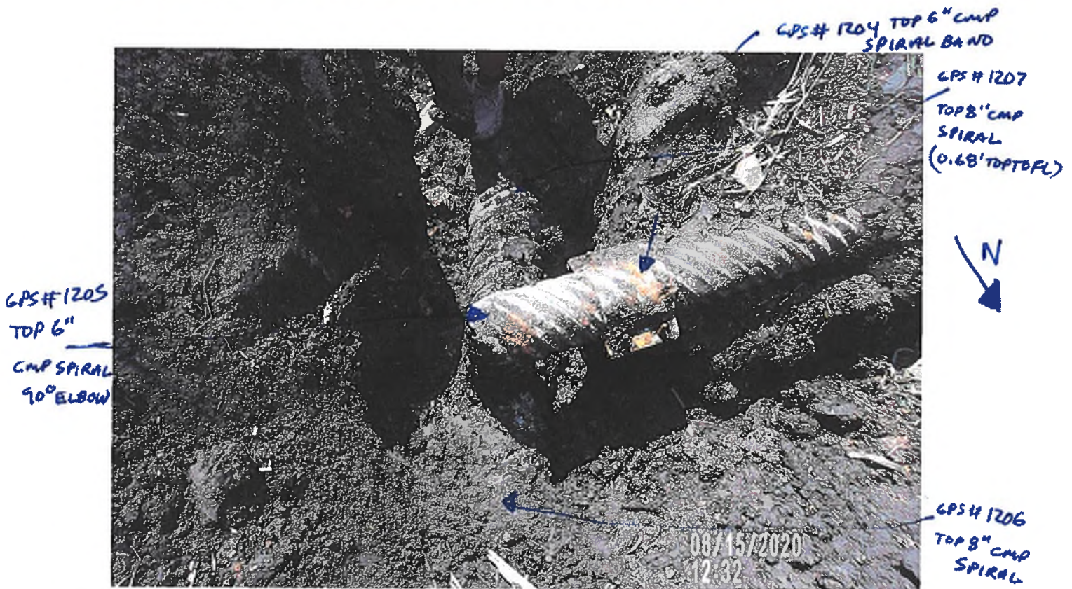
PICTURE # 3749 IS LOOKING SW AT 6" CMP SPIRAL FROM FIELD TIED INTO 8" CMP SPIRAL FROM BEEHIVE INTAKE AFTER BEEHIVE INTAKE HAS BEEN REMOVED
