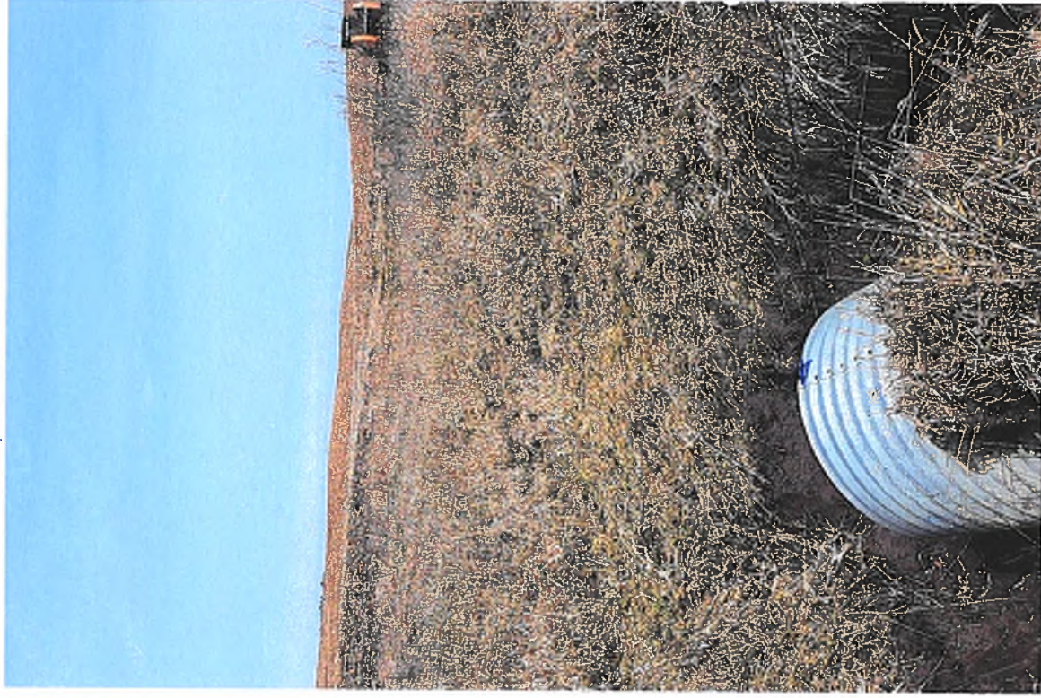
PICTURE #9 IS LOOKING NORTH OF 36" CMP SURFACE DRAIN INLET AT GRASS WATERWAY
