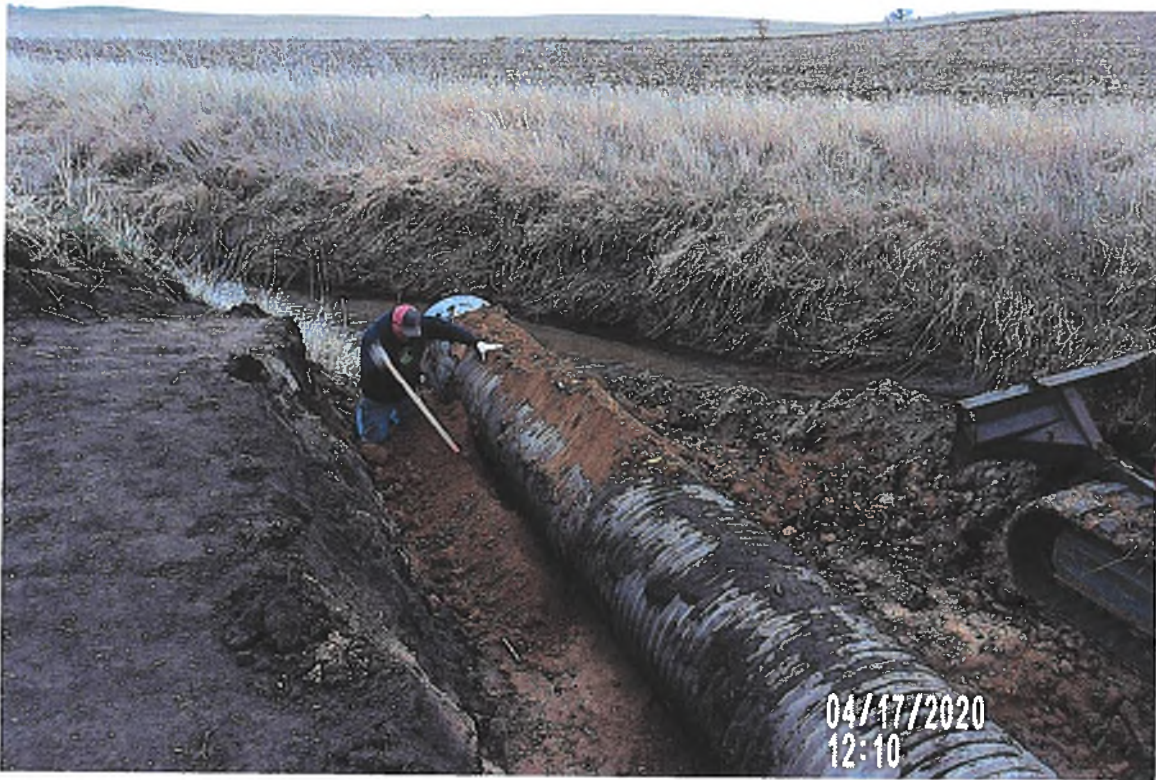
PICTURE #3380 IS LOOKING SW SHOWING CREW TAMPING IN BACKFILL SOIL UNDER HAUNCH OF CMP
