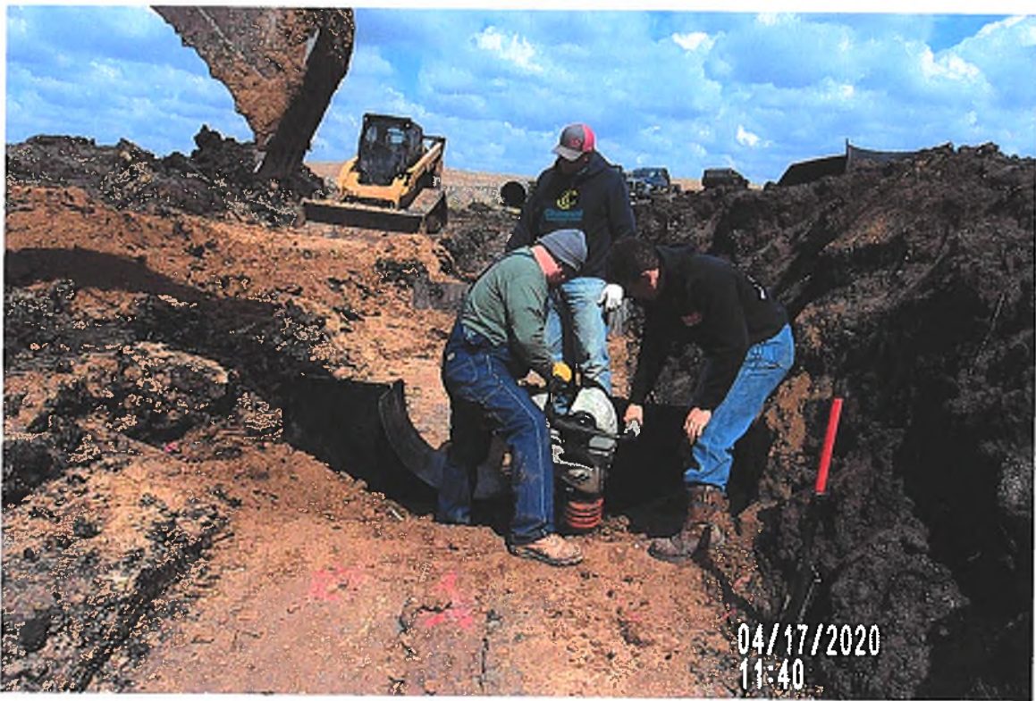
PICTURE # 3376 IS LOOKING NW SHOWING CREW VIBRATORY PLATE COMPACTING AROUND HDPE ANTISEEP COLLAR
