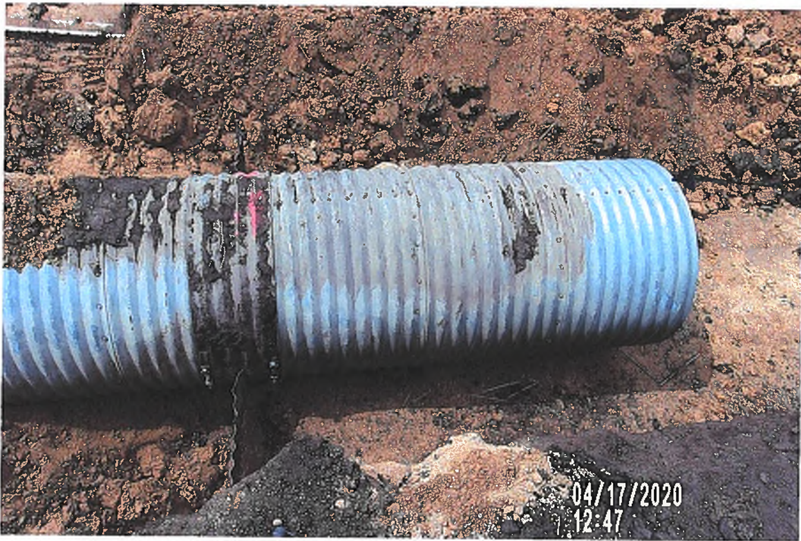
PICTURE# 3382 IS LOOKING SW SHOWING ORIGINAL CMP. ANTI SEEP COLLAR BOLTED ON 36" CMP 6.5' ± SE OF NORTH END OF 36" CMP SURFACE DRAIN.
