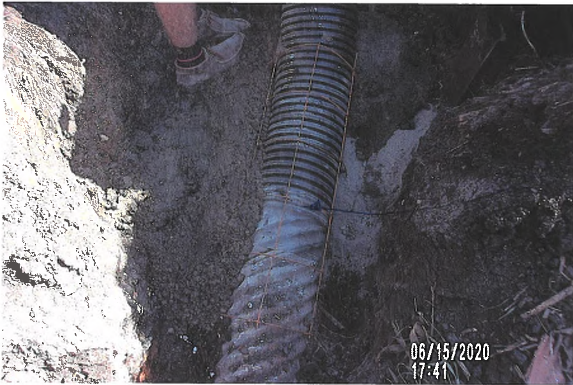
PICTURE # 3761 IS LOOKING SW SHOWING 1.5' X 2.5' 6" X 6" WIRE MESH AROUND CONNECTION BEFORE CONCRETE POURED
