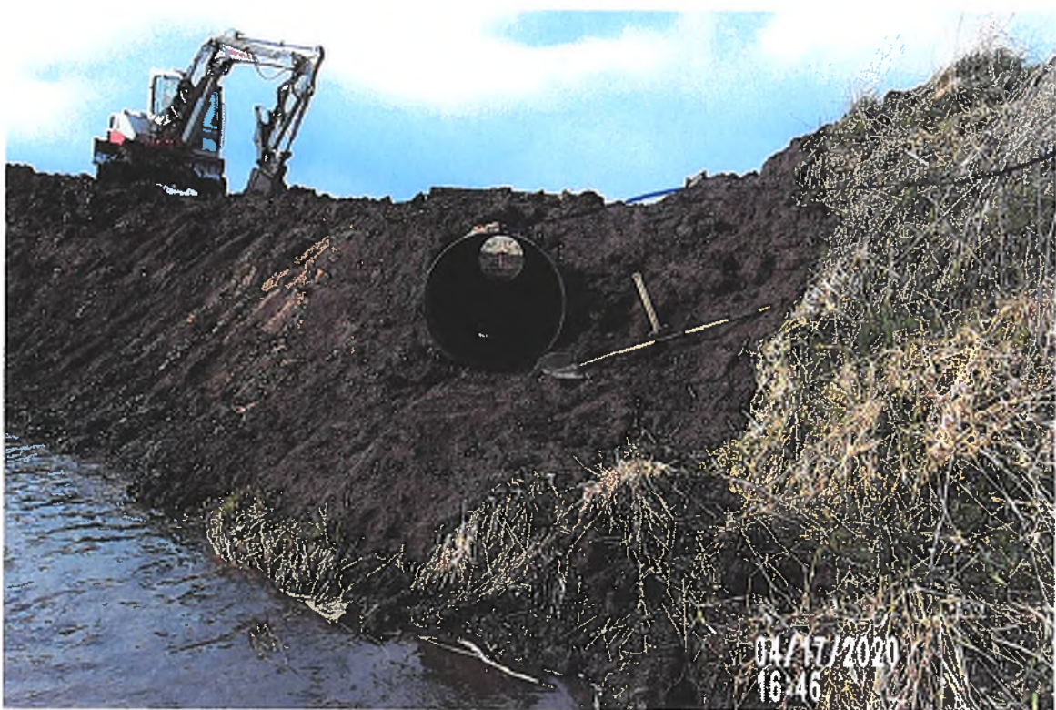
PICTURE# 3391 IS LOOKING NW AT DRAINAGE DITCH BANK GETTING BACK FILLED AROUND 36" CMP SURFACE DRAIN.
