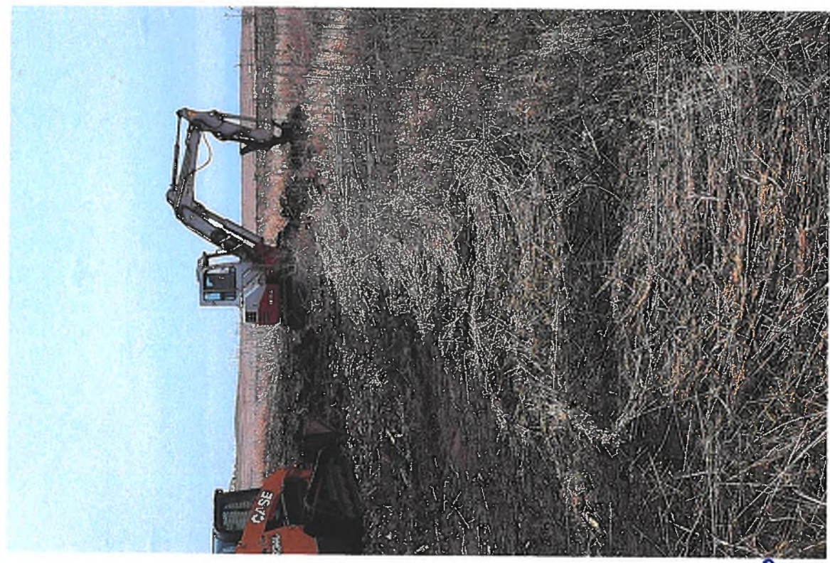
PICTURE #10 IS LOOKING SOUTH SHOWING GREW STRIPING OFF TOPSOIL FROM AROUND 36" CMP SURFACE DRAIN
