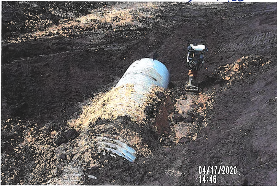
PICTURE# 3390 IS LOOKING NW SHOWING CREW STILL JUMPING JACK COMPACTING BACKFILL SOIL ON NORTH END OF 36" CMP SURFACE DRAIN. / GPS#428
