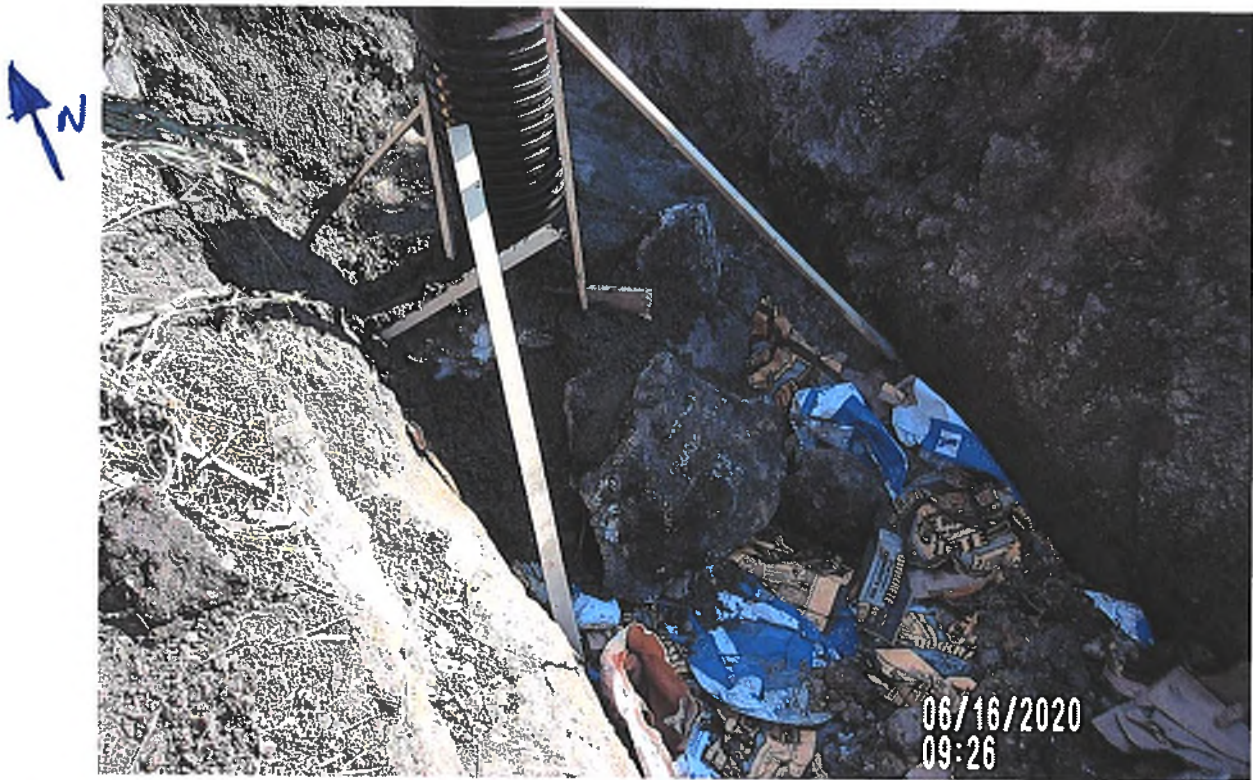
PICTURE # 3767 IS LOOKING NE SHOWING OLD CONCRETE CHUNKS CONCRETED IN TO SUPPORT 8" SW HOPE PERF TILE FOR 8" HICKEN BOTTOM INTAKE.
