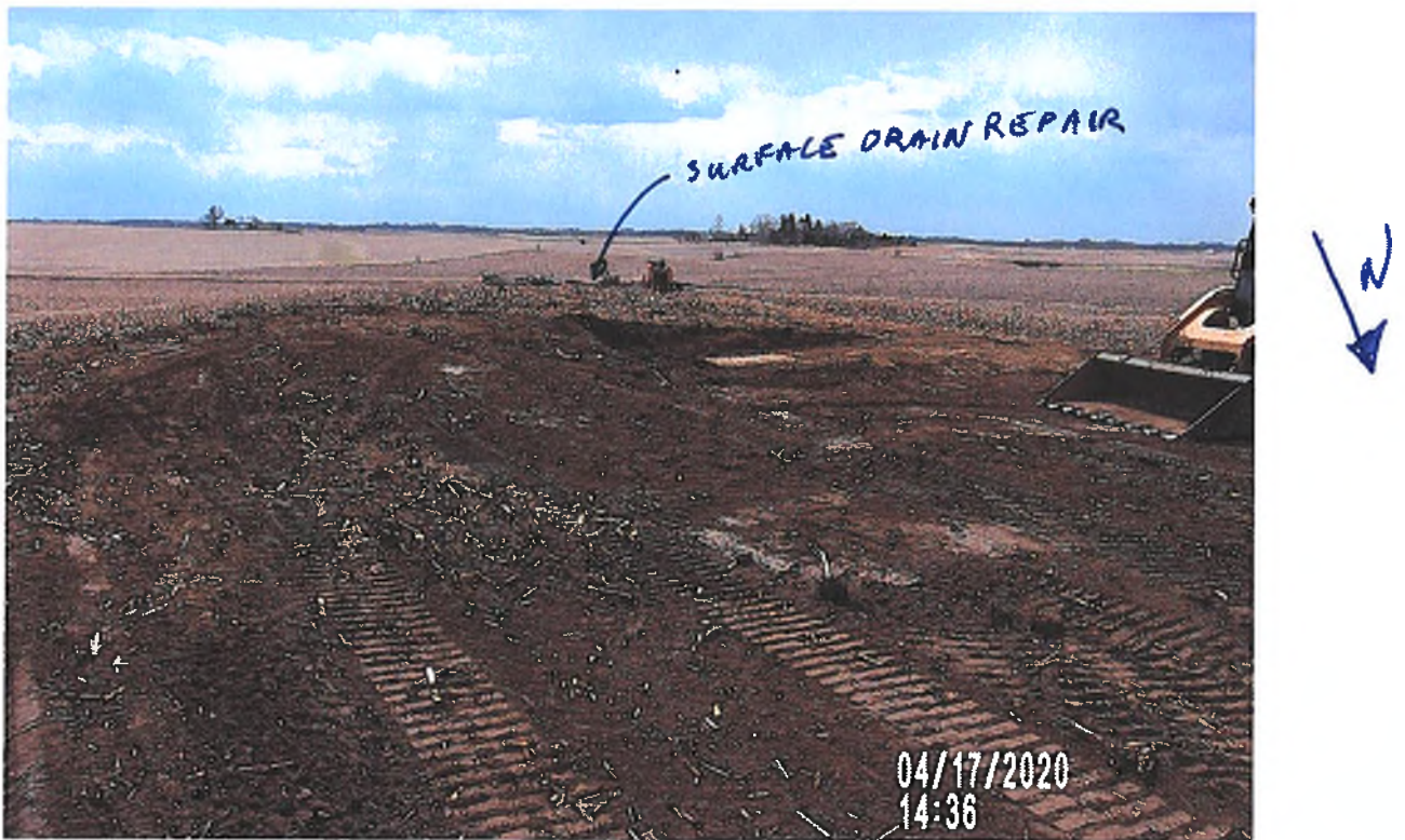
PICTURE # 3389 IS LOOKING SW FROM BORROW AREA TO CMP SURFACE DRAIN REPAIR ABOUT 713.6' TO SW
