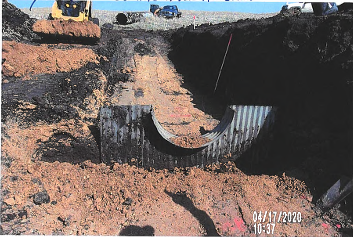
PICTURE # 3373 IS LOOKING NORTH SHOWING CREW HAVING ORIGINAL METAL ANTISEEP COLLAR IN PLACE (7.0' SE OF NORTH END OF CMP SURFACE DRAIN). CREW HAULING IN LIMY CLAY SOIL TO BACKFILL AROUND ANTISEEP COLLAR.
